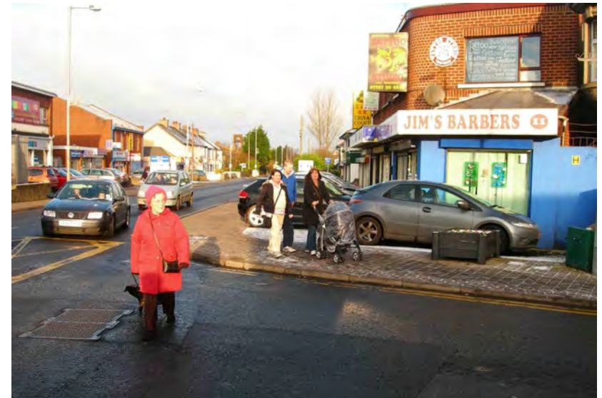
Figure 2.10: No dropped kerb at Portland Avenue makes walking difficult for some users
