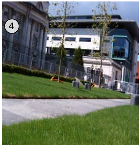
Construction of a new publicly accessible pedestrian realm between Belfast's Law Courts is underway. This space will transform the east-west city axis, creating a physical and visual connection with the riverside.
