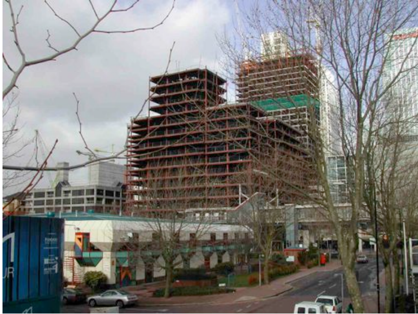
Millharbour – first generation low-rise offices about to make way for marching towers
