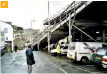
The town centre car park is an unsightly and unsound structure
