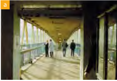
Important bridge link over tracks from station, but outworn and unpleasant
